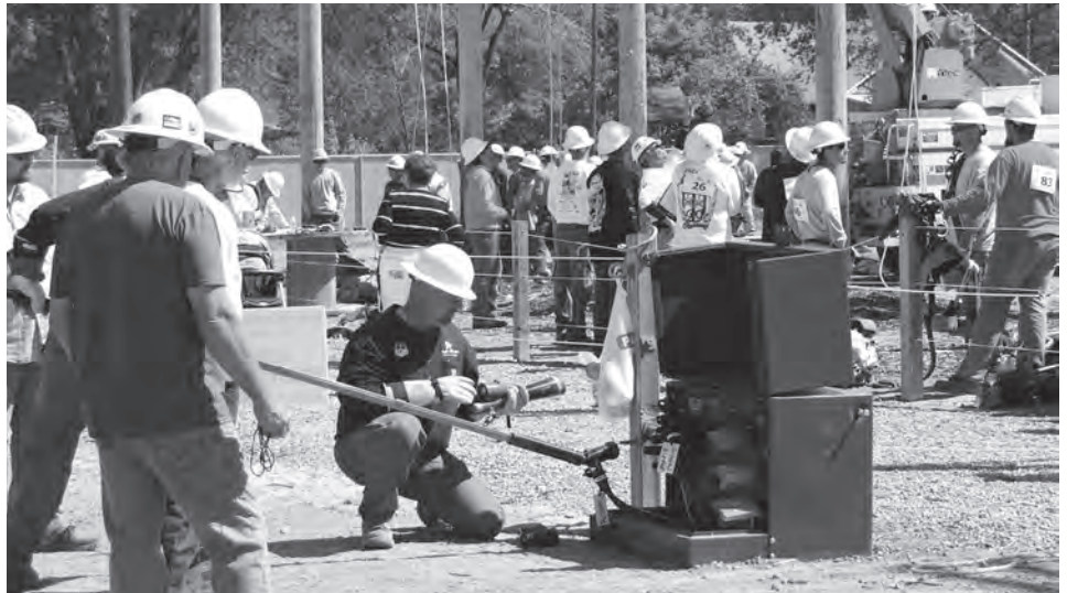
Lineman Curtis Berg prepares to replace a “blown fuse” during one of the Utah Lineman Rodeo events.
